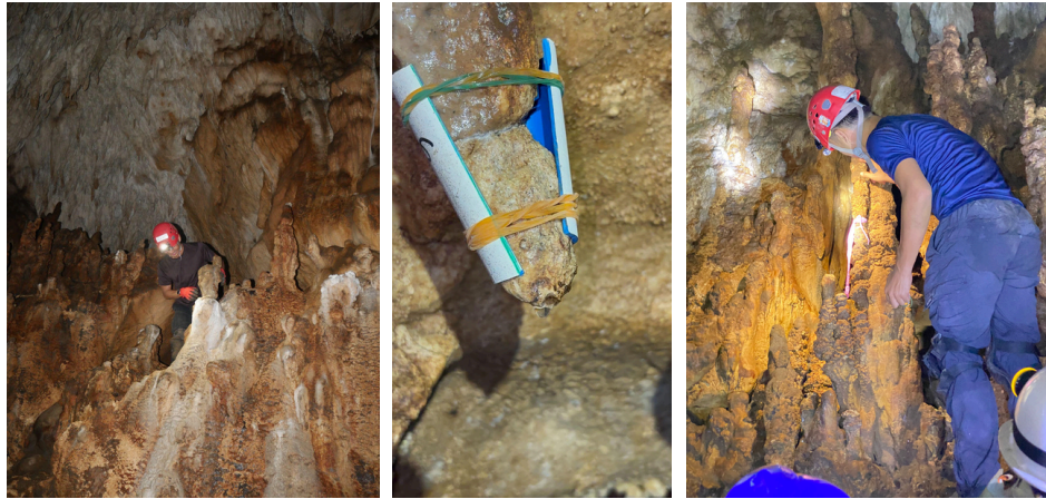
Speleothem repair conducted in accordance with established conservation protocols adapted from the techniques of Michel Mansur of the Cave Formation Repair Project. Photo: Neena Rachel Marie Panal.
