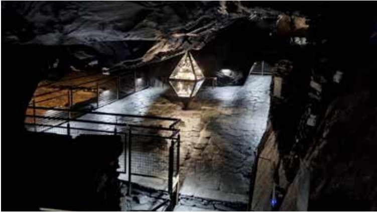
The exit passage at Martelange mine includes GVA PIXELDOME luminaires.
